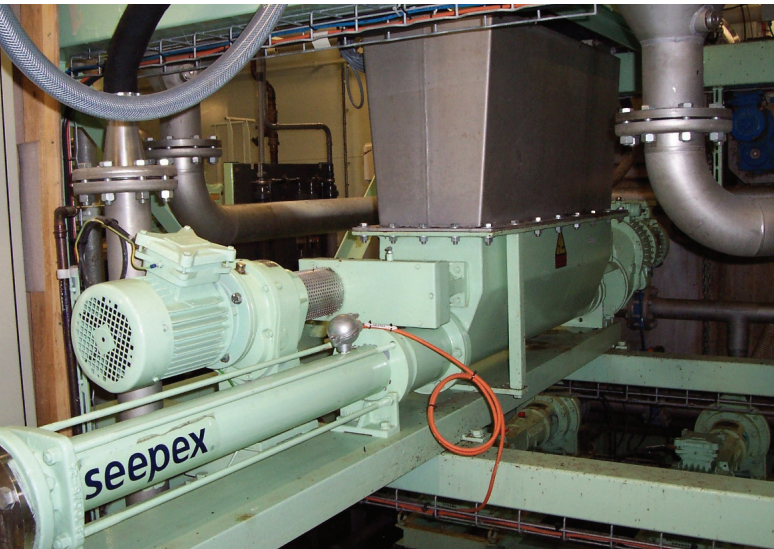
seepex pump of range BTI for conveying dewatered sludge into the drier
