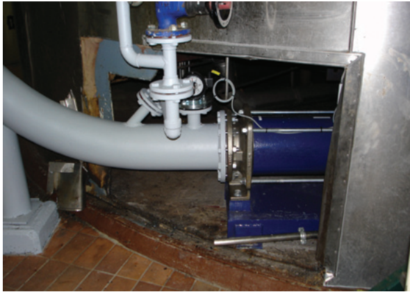
seepex BT open hopper pump replaced expeller unit, installed under lauter tun
