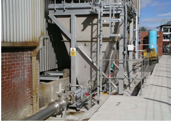
The final engineered installed solution
