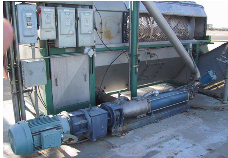
seepex Pump with TSE dry run protection receives gravity fed, de-stemmed berries on their way to processing tanks.
