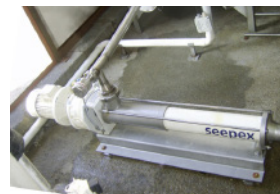
Installed seepex pump BCSO
