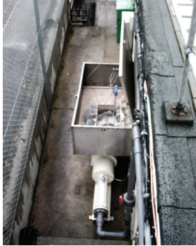
seepex BTH range pump mounted outdoors against the wall of the production area
