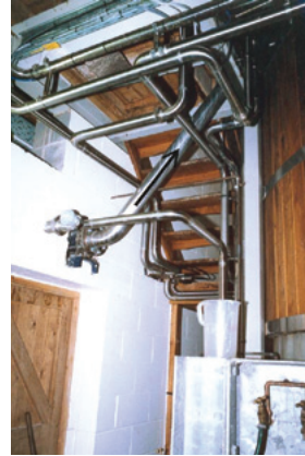
Grist case/miller outlet below mash tun, seepex pump transporting mixed grain and hot water back up into mash tun
