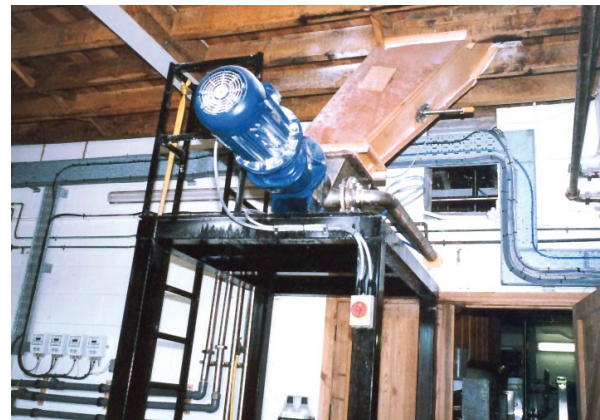
seepex pump installed underneath grist case, receiving milled grain and mixing with hot water
