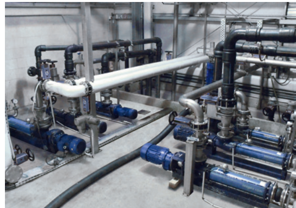
Six of the total of eleven seepex pumps at the biogas plant in Werlte
