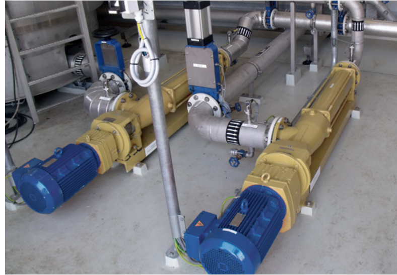
Two of five seepex BN range pumps at the Watershap biogas plant
