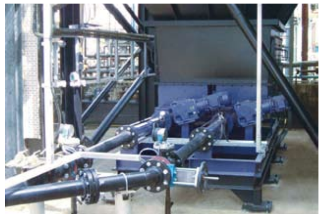
Pumps of range BTEI 17-24 installed under reception silo Conveying product: Oily sludge cake with a ds content of 60 % Conveying capacity: 4 m 3 /h (17 GPM) • Pressure: 16 bar (232 PSI) Temperature: 5 – 40 °C (41 – 104 °F)
