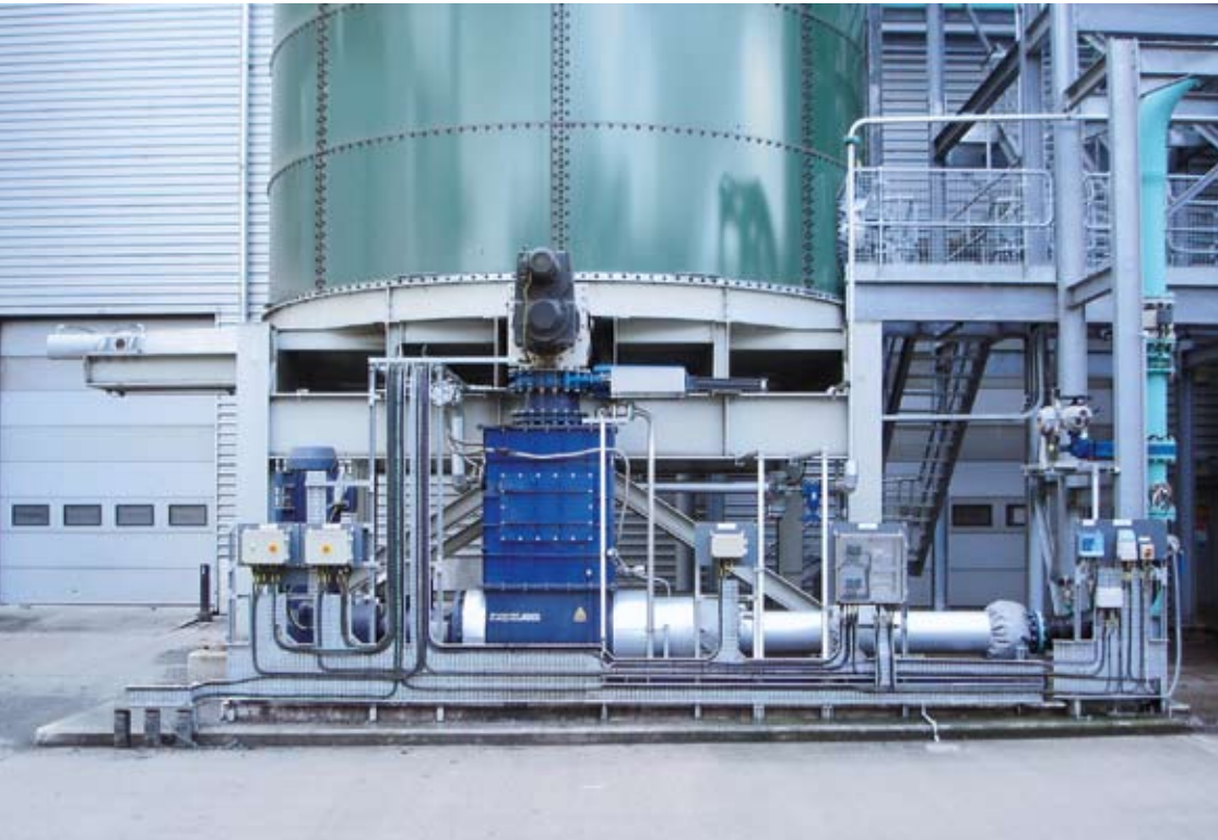
seepex pump with numerous controls: motor control, dry running protection (TSE), over pressure control and level control via load cells.
